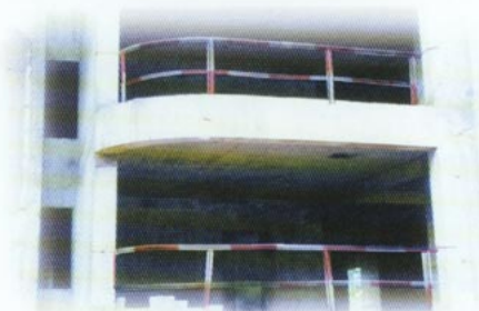
阳台临边防护
